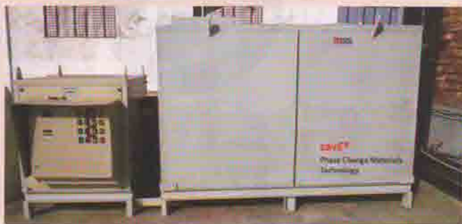
Figure 6: 40 TRH flat plate TES system installation with a 6 TR chiller
